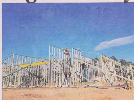
BUILD UP. Construction has begun on the South East Regional Hospital carers accommodation. Picture: Lynne Koerbin
